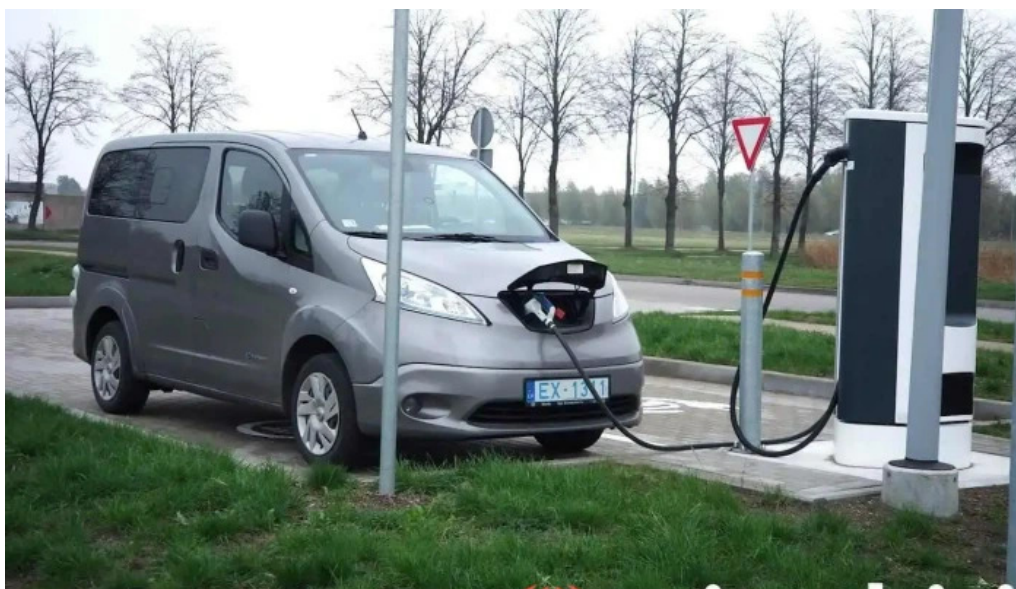
Csdd charging station liepāja
