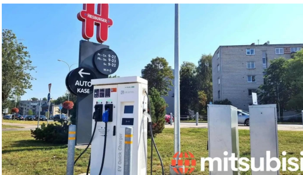
Csdd charging station j?rmala
