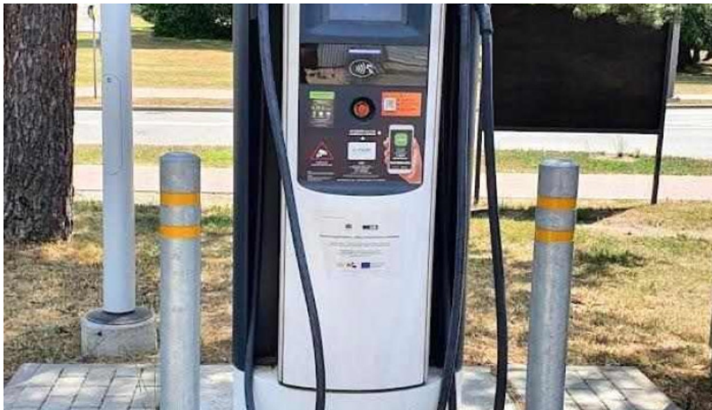
Csdd charging station ikšīle
