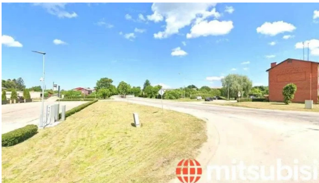
Csdd charging station dundaga
